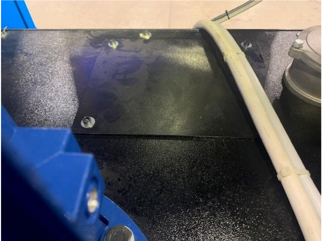
(Access panel, top lid of tank)
